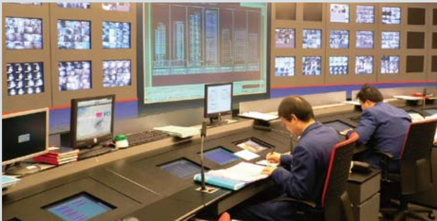
Modern commercial buildings are monitored by computerized building management system.
