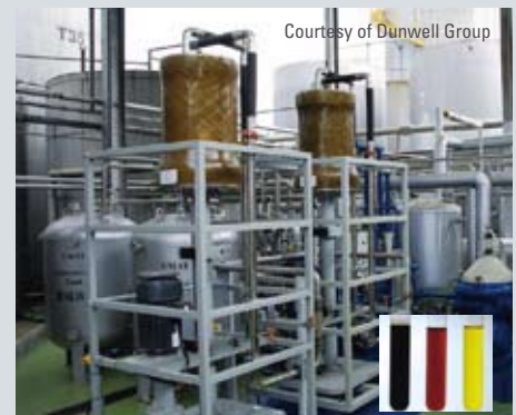
Vibratory membrane recycling system for used oil. The small photo shows the oil at different filtering stages.
