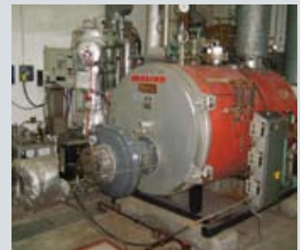
An industrial boiler in Thermal Laboratory.
