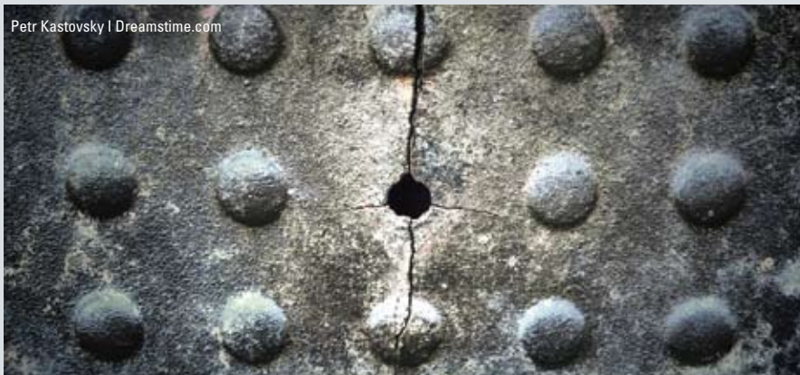
Cracks emerging from a rivet hole which can be found in many metallic structures.
