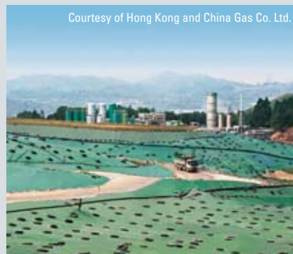
The landfill gas plant in the The North-East New Territories Landfill at Ta Kwu Ling. The plant is expected to supply over 10,000 m 3 /hr of methane in 2015.
